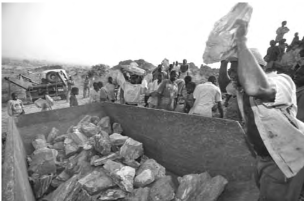
Peasants building a stone wall near Kongoussie, Burkina Faso, to reduce erosion. © Knut Mueller/Das Fotoarchiv.
