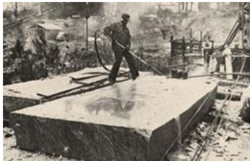
A worker uses a special burner to finish a slab of Pyramid Blue granite. Photo: Courtesy of Fendley Enterprises Inc.
